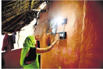
Offgrid Power supply
